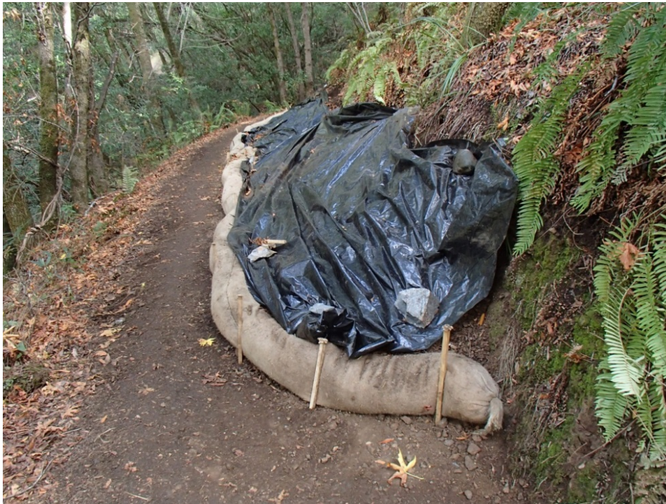
Photo 27.3 - Excavated Soil Retained by Straw Wattles and Covered to Protected from Erosion
